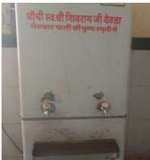
Figure 2: Water Cooler at a facility in Pali District
