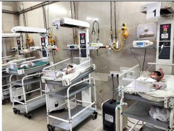
SNCU ward, DWH, Gonda
